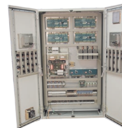
Control cabinet for generator management
